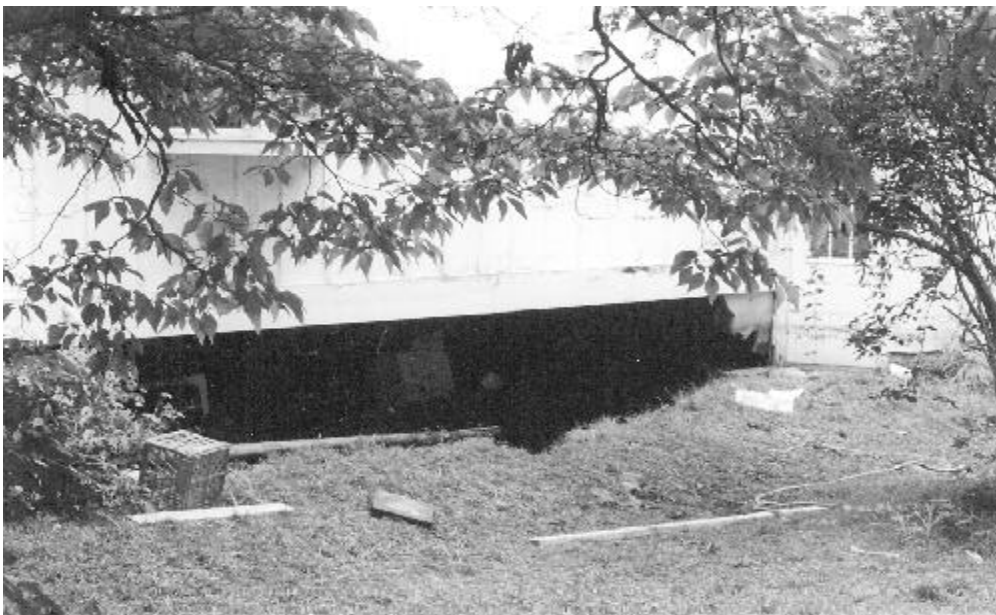
The heavy rains on August 10 and 11 took out the foundation of this house on Sherier Place and Macomb and caused serious damage to other Sherier Place and neighboring homes.
