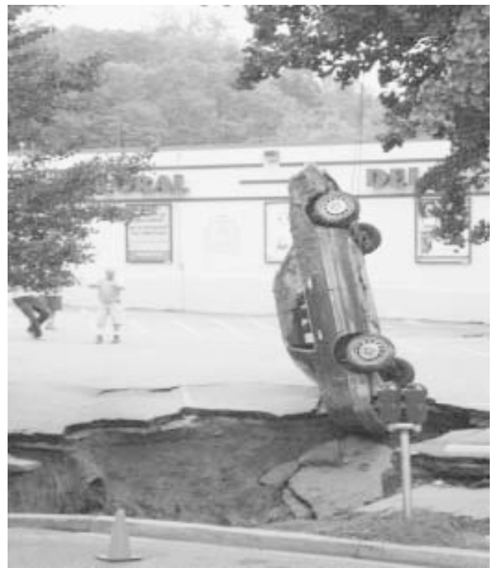
After weeks of hot and dry summer weather, the rains came August 10 and 11 and did much damage to many homes and businesses throughout the District, but seemed to hit the Palisades particularly hard. A sinkhole in the MacArthur Safeway parking lot caused by the rains literally swallowed up a car, being removed here. Photo by Jim Wheeler.
